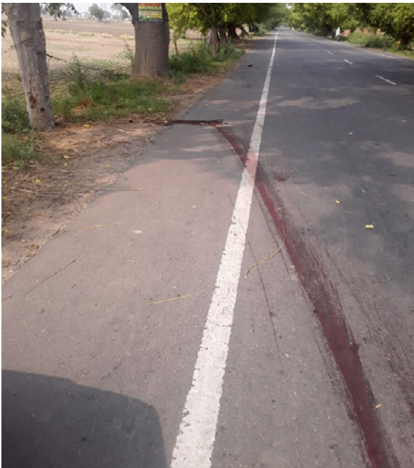
Image 2: Photograph of the scene of accident.
